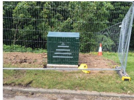
13b New gas meter housing
